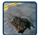
POTHOLES/ DAMAGED PAVEMENT
